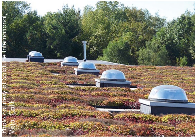
Bell's® Brewery Inc., Galesburg, Mich., integrated a daylighting system into the building's vegetative roof.
