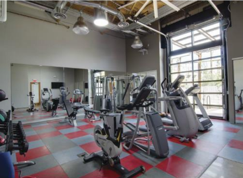
ABOVE: An expansive gym and locker room are efficiently heated and cooled using state-of-the-art “green” technology.
